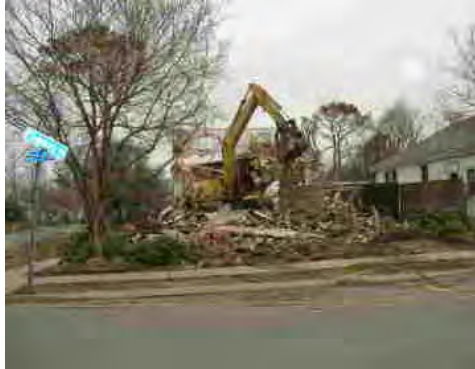
Owner was watching her house being leveled. She said that she was going to rebuild.
