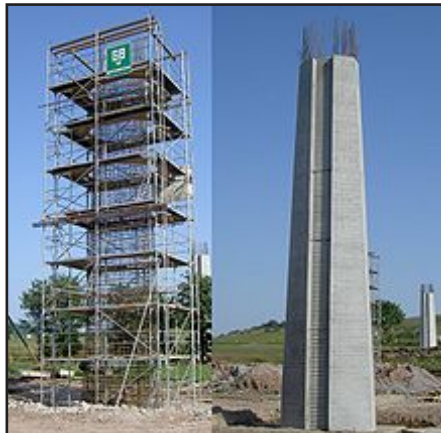
Here is a reinforced concrete column, seen before and after the concrete has been cast in place around the rebar cage.
